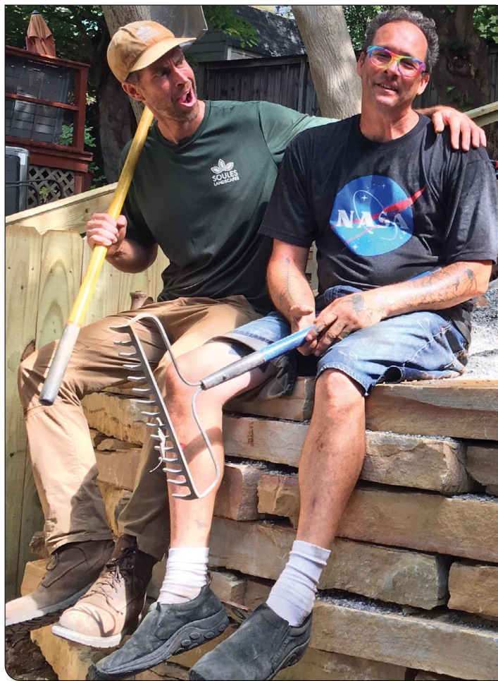
Hudson Souls and The Good Reverend David DeChant building the new retaining wall (and everything else) at Little's ShadeTree.
