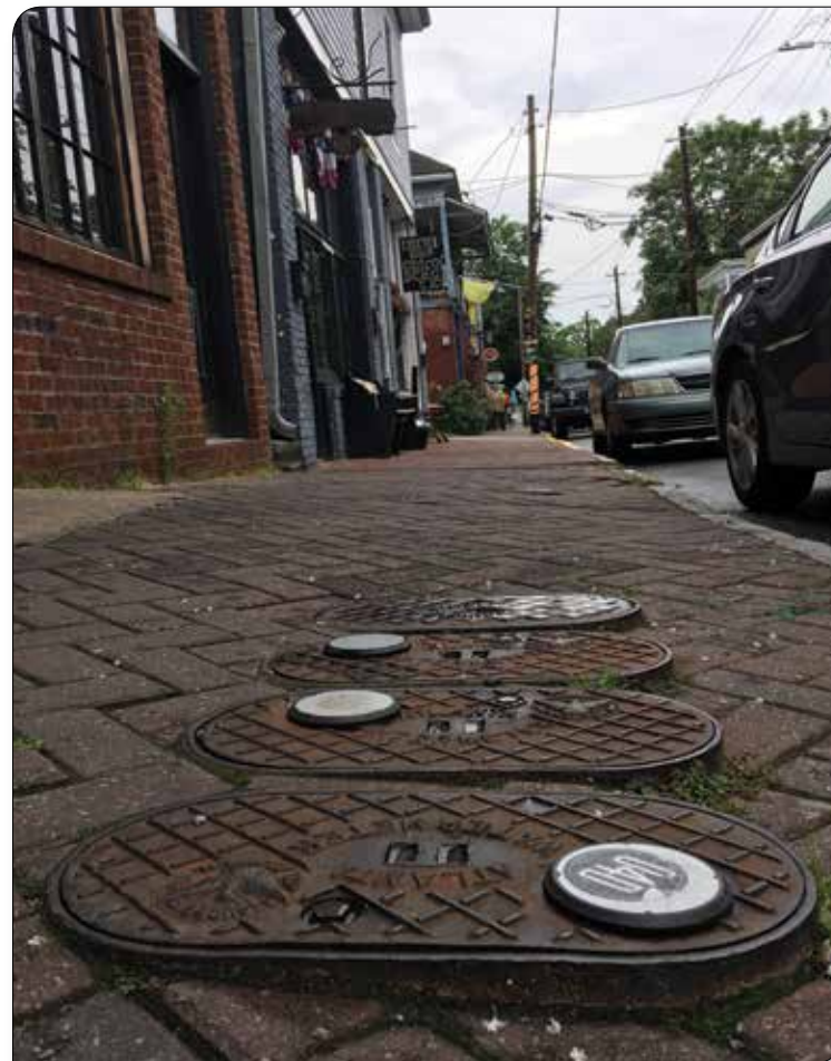
Water meter covers on Carroll Street.
